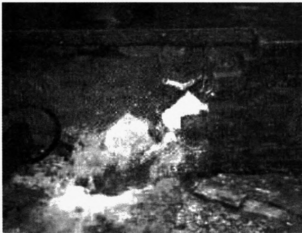
Figure 8 - Brickwork wall broken by flood water, Malton, U.K., November 2000 (Kelman and Spence [22])
