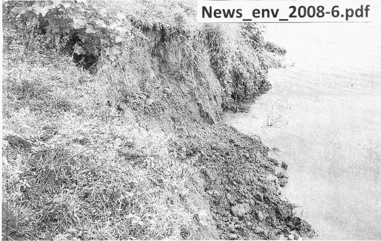
The damaged section of the dam
