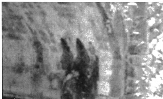
Figure 6: Seepage through blocks
