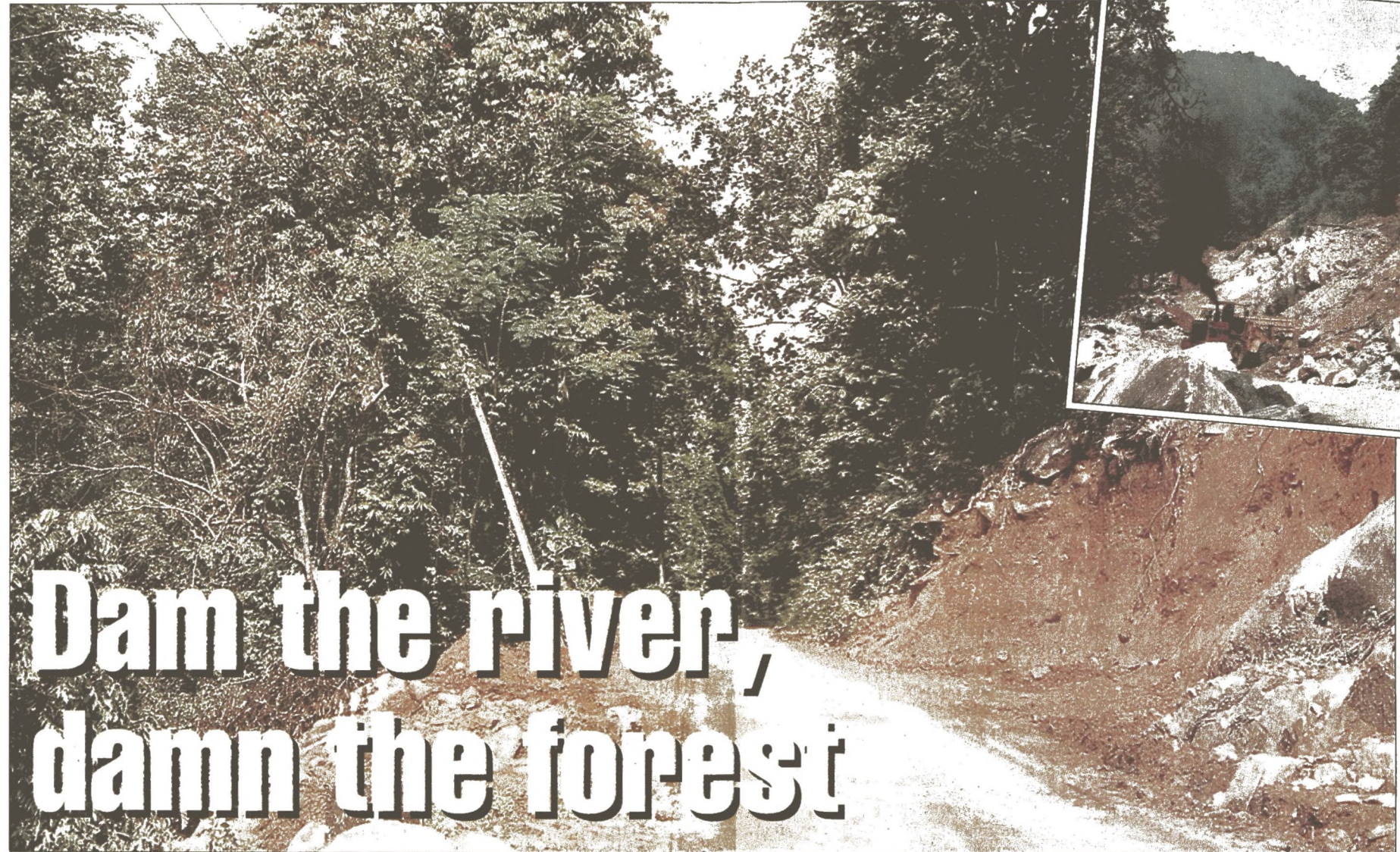
Road widening: Not mentioned in the EIA that such massive clearing would take place
