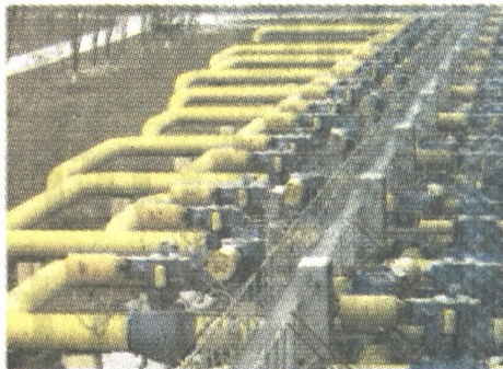
Gas storage and transit point in Boyarka, just outside Kiev in Ukraine
