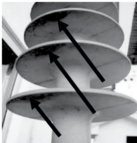
Figure 3 - Collected dirt at under side of insulator #F
