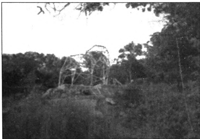
Figure 9: View of the collapsed stage of the tower
