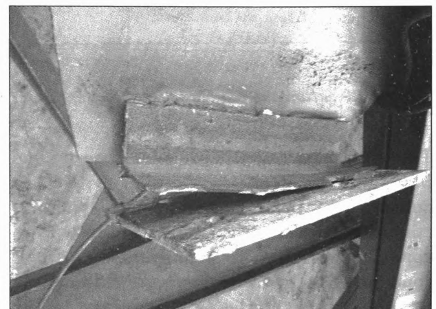
Figure 8. Poor Connection at Shoe Plate
