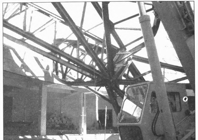
Figure 6. Collapsed truss system
