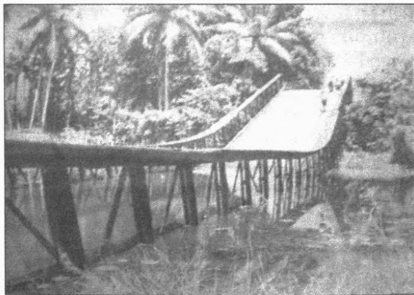
Figure 1: Failed bridge at Paragastota
