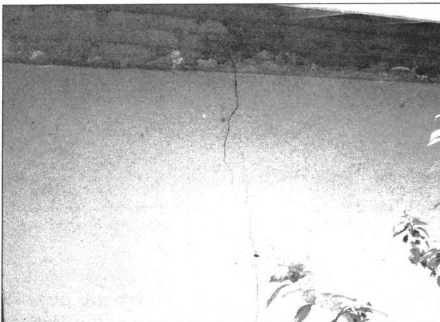
Figure 3: Shrinkage cracks of the walls of a house made out of cement Stabilized Soil Blocks in Matara
