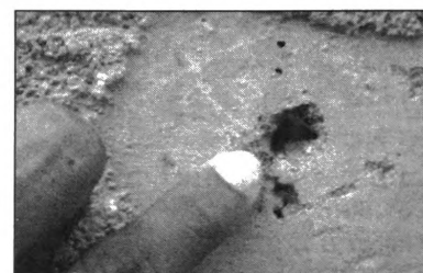
Figure 6: A defect on an un-stabilized soil block wall of a house in Kosgama-Avissawella
